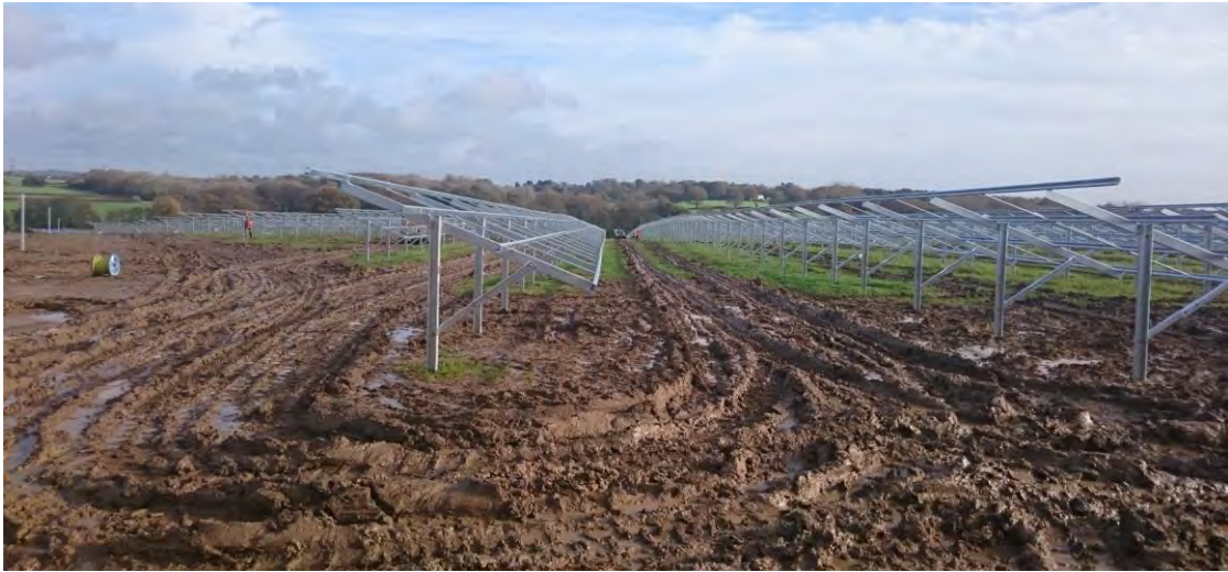
Inserts 37 and 38: Winter Installation (2015) and Operational Site (2022)
